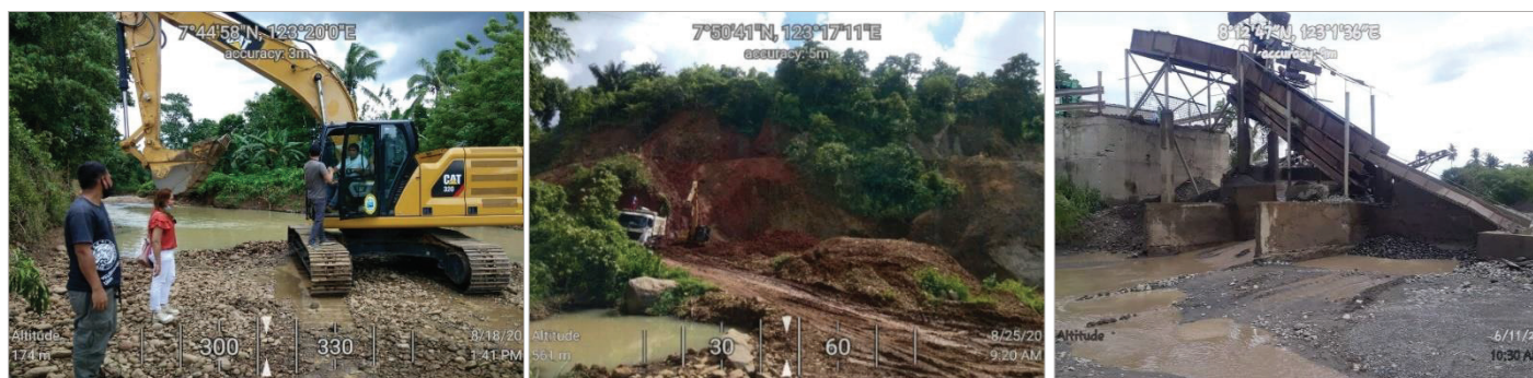
Figure 9.4 Several investigations were conducted in Region 9, relative to the implementation of responsible mining in the country e.g. inspection and investigation of sand (left); mountain quarrying (middle); and use of heavy equipment in sand and gravel quarrying (right)
