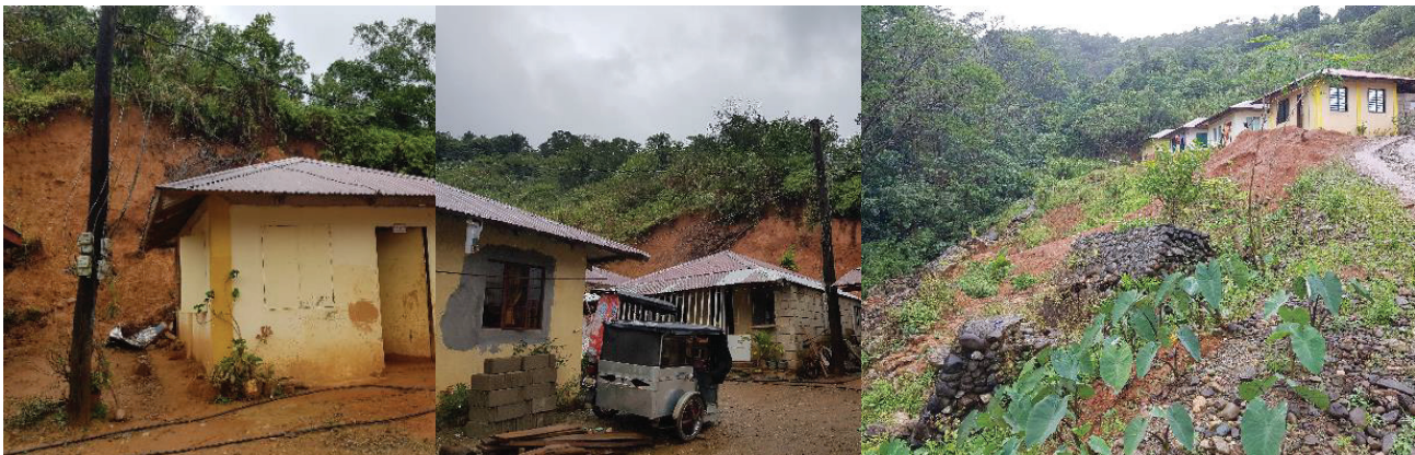
Figure 9.1 Weak and loose slope materials affected several households due to excess surface run-off in Star Village in Region 2.
