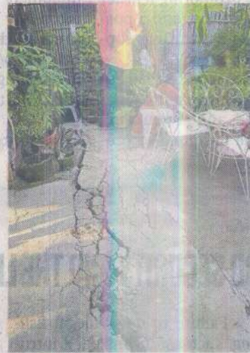
CRACKS Ground fissures, as shown in this photo taken on May 12, threaten at least 10 houses in San Carlos City, Negros Occidental. —PHOTO COURTESY OF THE SAN CARLOS CITY DISASTER RISK REDUCTION MANAGEMENT OFFICE
