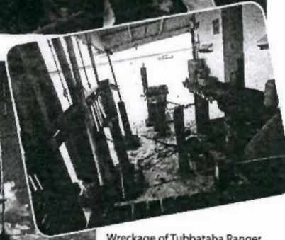
Wreckage of Tubbataha Ranger Station after December weather disturbance
