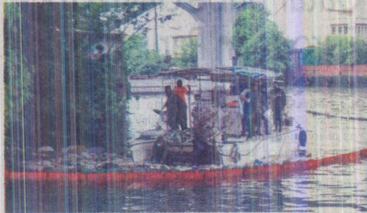
■ Volunteers from the Philippine Coast Guard install floating trash barriers. CONTRIBUTED PHOTO
