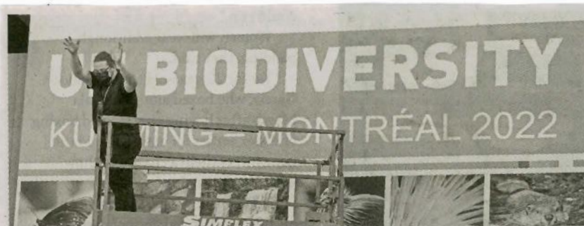
WORKERS set up the Montreal Convention Centre on December 2 in preparation for the COP15 UN conference on biodiversity in Montreal. Environmental leaders are gathering in Montreal to hammer out a framework they hope will help provide much-needed protection for the world's biodiversity. PAUL CHIASSON/THE CANADIAN PRESS VIA AP
