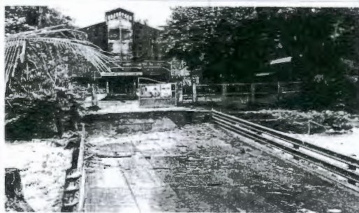
COLLAPSE A bridge leading to the town center of Malalag, Davao del Sur, collapses on Thursday due to the strong river current amid widespread flooding, in this photo taken on the same day.
