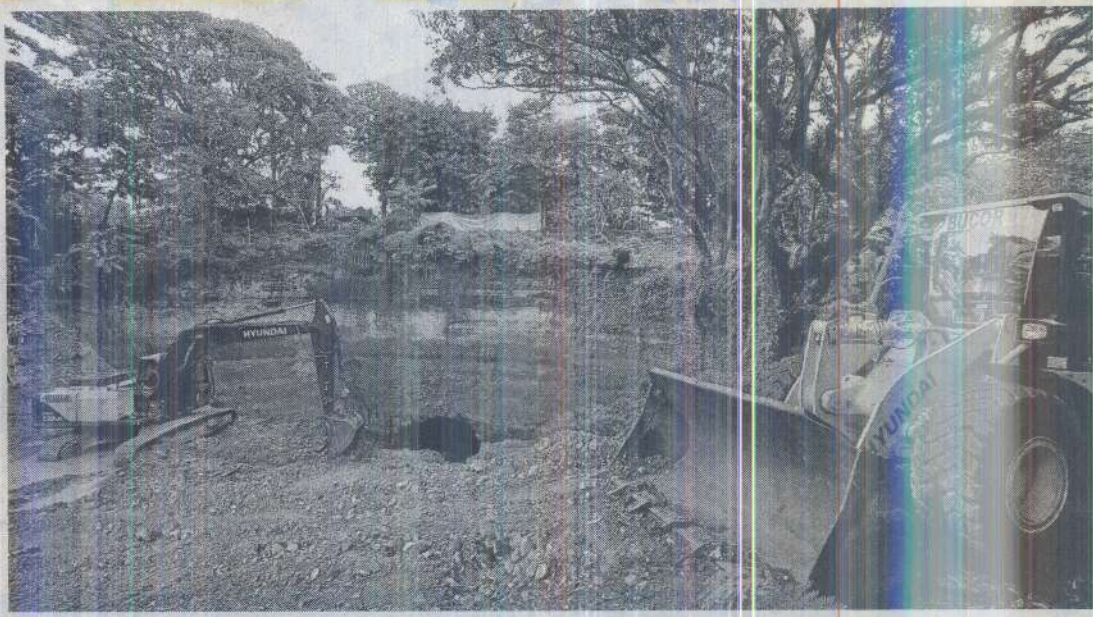
DEEPEST DIG The "tunnel" built in what suspended corrections chief Gerald Bantag said was to have been part of a diving pool could be seen at the bottom of a rock wall at the deepest site within a 4-hectare excavation area inside the New Bilibid Prison reservation. —RICHARD A. REYES
